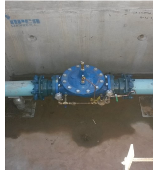
One of fourteen pressure reducing stations
